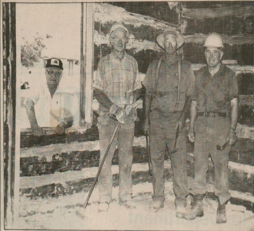
Ross Code watches looks through the window of the house in which he was born as workers dismantle the building for re-location to Forester's Falls as the new Ross Township Historical Society museum. Workers, from left, are Doug Patterson, Mac Coughlin, and Bill Oates.
